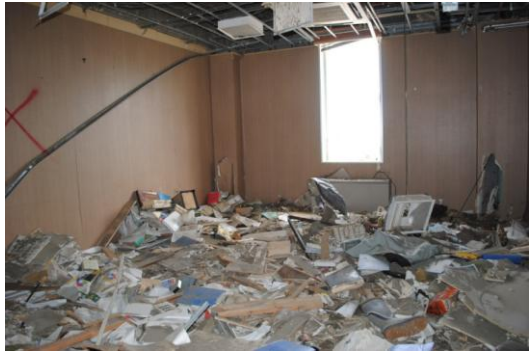
Records scattered across the floor inside the the tsunami-ravaged city hall building.
